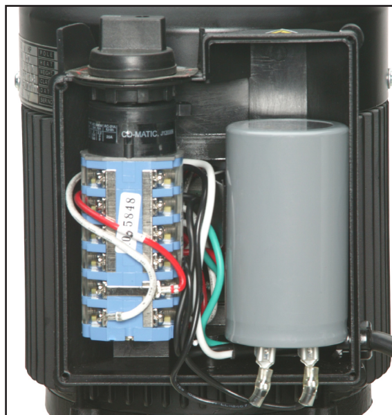
Figure 19. Motor switch and capacitor (front view).
